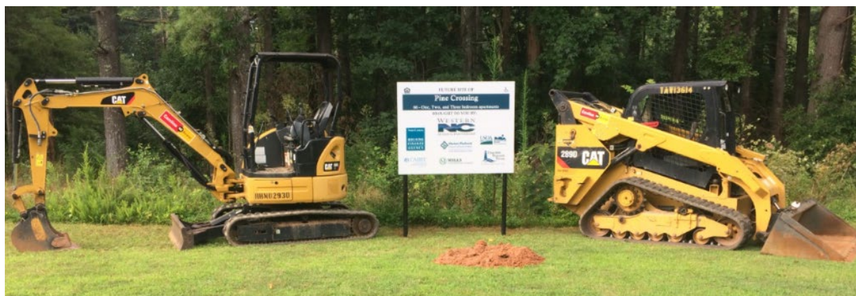
Photo 1: Breaking ground on Pine Crossing, a 66 unit, multifamily housing development in Valdese, NC
